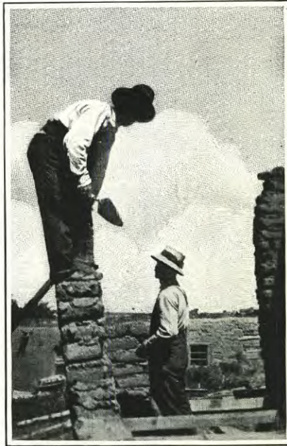
THE WALL THAT BUCKLED
